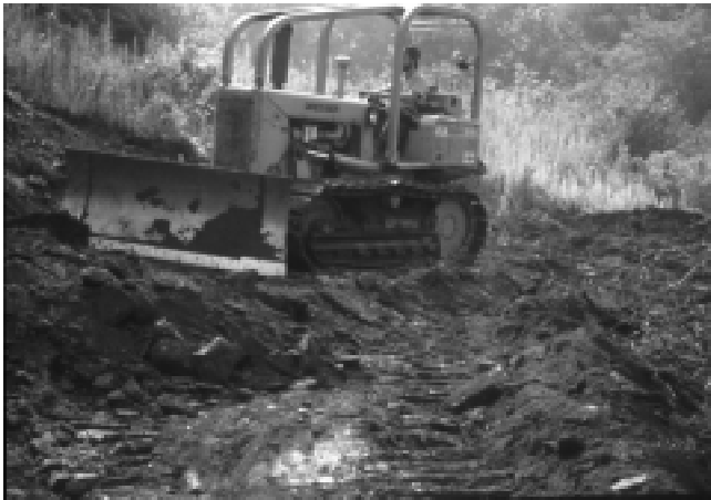
Figure 5. Using large equipment for site preparation is efficient but is not suitable for all areas.
