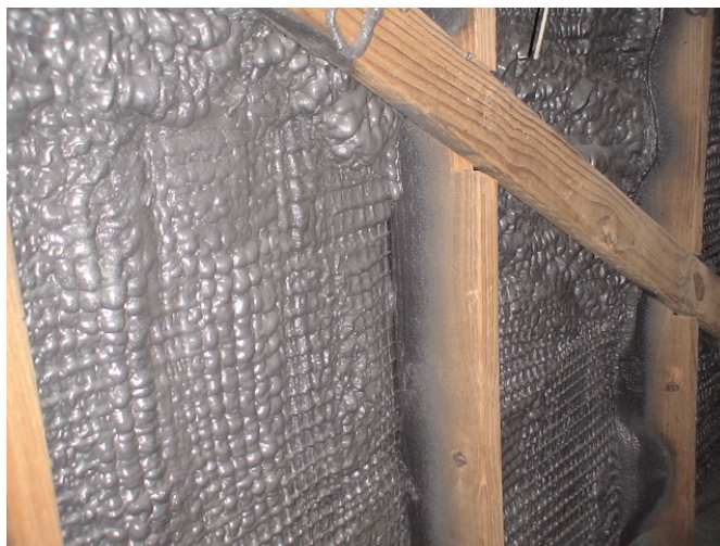
Figure 2. A curtain-sided wall converted to a solid wall by spraying foam insulation. (Courtesy: M. Czarick, Univ. of Georgia)
