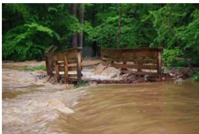
The new bridge to Weston Manor took a beating during a springtime storm.
